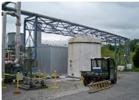
Figure 3.16. The Chromium Water Treatment System
