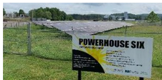
Figure 3.4. Oak Ridge Powerhouse Six Solar Farm
